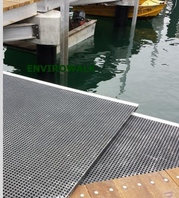
EnviroTread custom safety Landing panels Darling Harbour, Sydney
